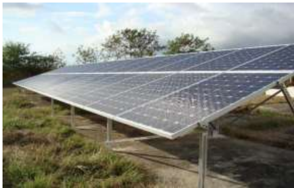
Figure 1. 7.5 kWp photovoltaic generator installed in SERC.
